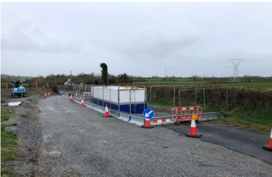
Image 4.24: Example of a Joint Bay Shelter
