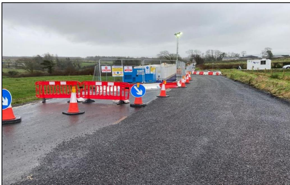
Image 4.4: Example of a Passing Bay (Ensuring Road Traffic Continues Around a Working Area)
